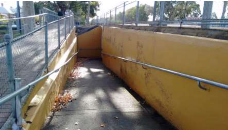
Photo 4. Down to underpass. Towards the platform (upper ramp). The street is at the left.
