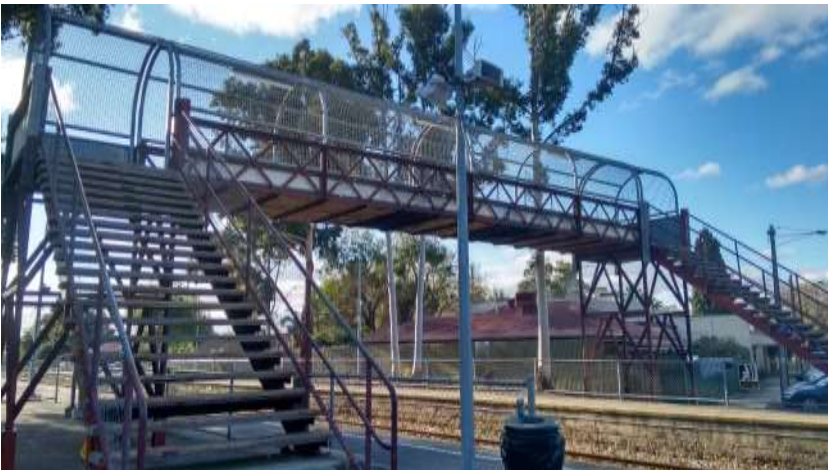
Photo 6. Sturdy and safe footbridge but the paintwork is slapdash. Minimal effort at maintenance.
