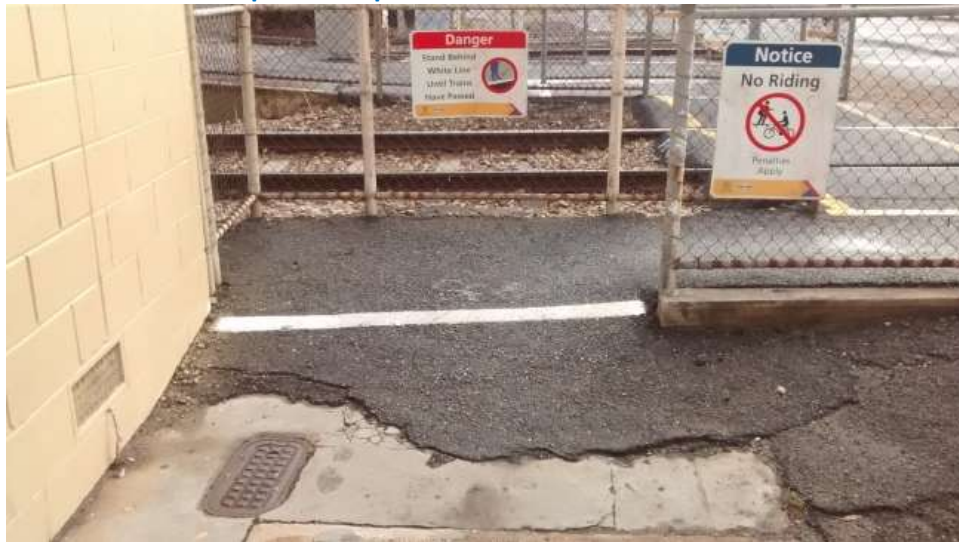
Photo 8. North East path disrepair
