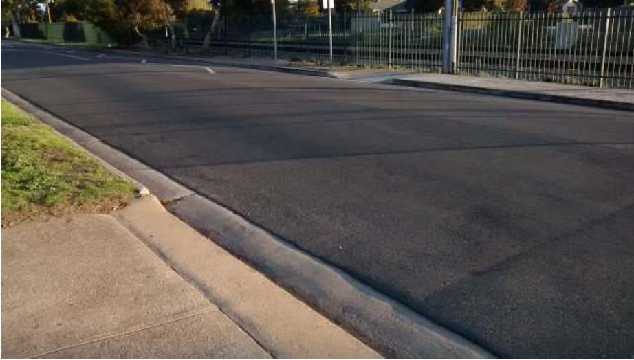
Photo 9. Gap in path
