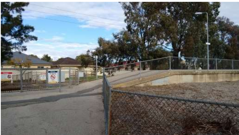
Photo 7. Cracked, steep and lopsided ramp
