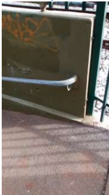
Photo 11. Very low handrail
